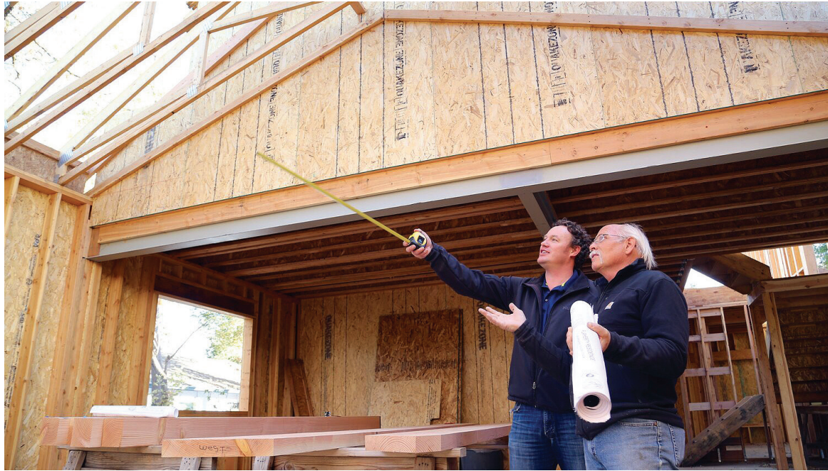
Skycastle's Head of design/build, Brandon David, discusses a framing detail with Site Supervisor Tim Hoefling.
